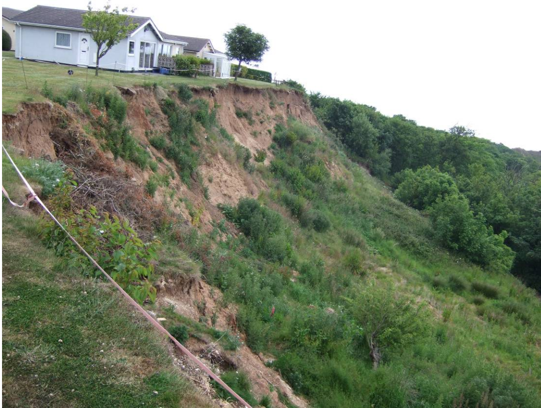
Plate 17 Cliff recession at Knipe Point Headland looking east (17 th June 2011)
