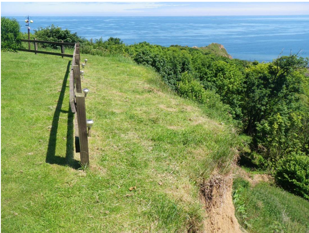
Plate 10 Cliff recession at Knipe Point Headscarp looking east (17 th June 2010)
