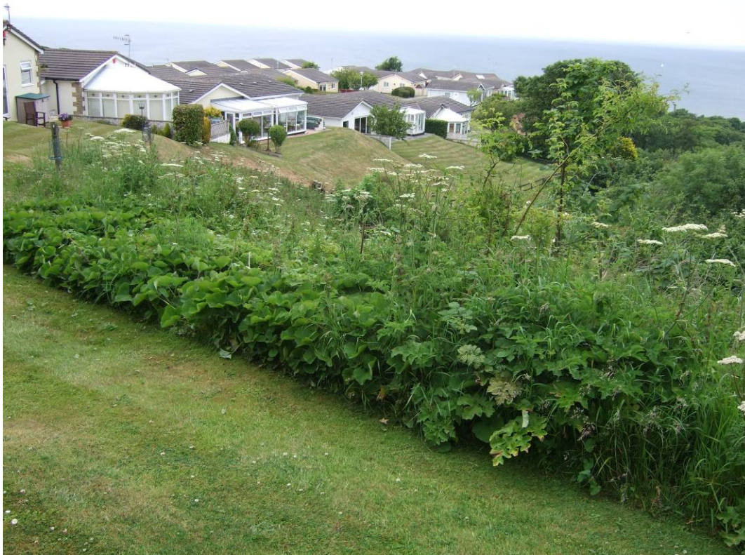
Plate 20 Cliff recession at Knipe Point Headland looking east (17 th June 2011)
